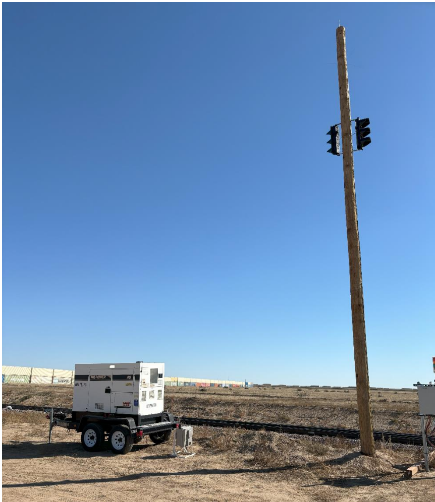
Figure 6-7 Outdoor Wayside Contention System Installation
